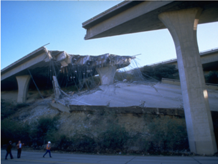
Damaged portion of the Golden State Freeway at Gavin Canyon, January 17, 1994.
