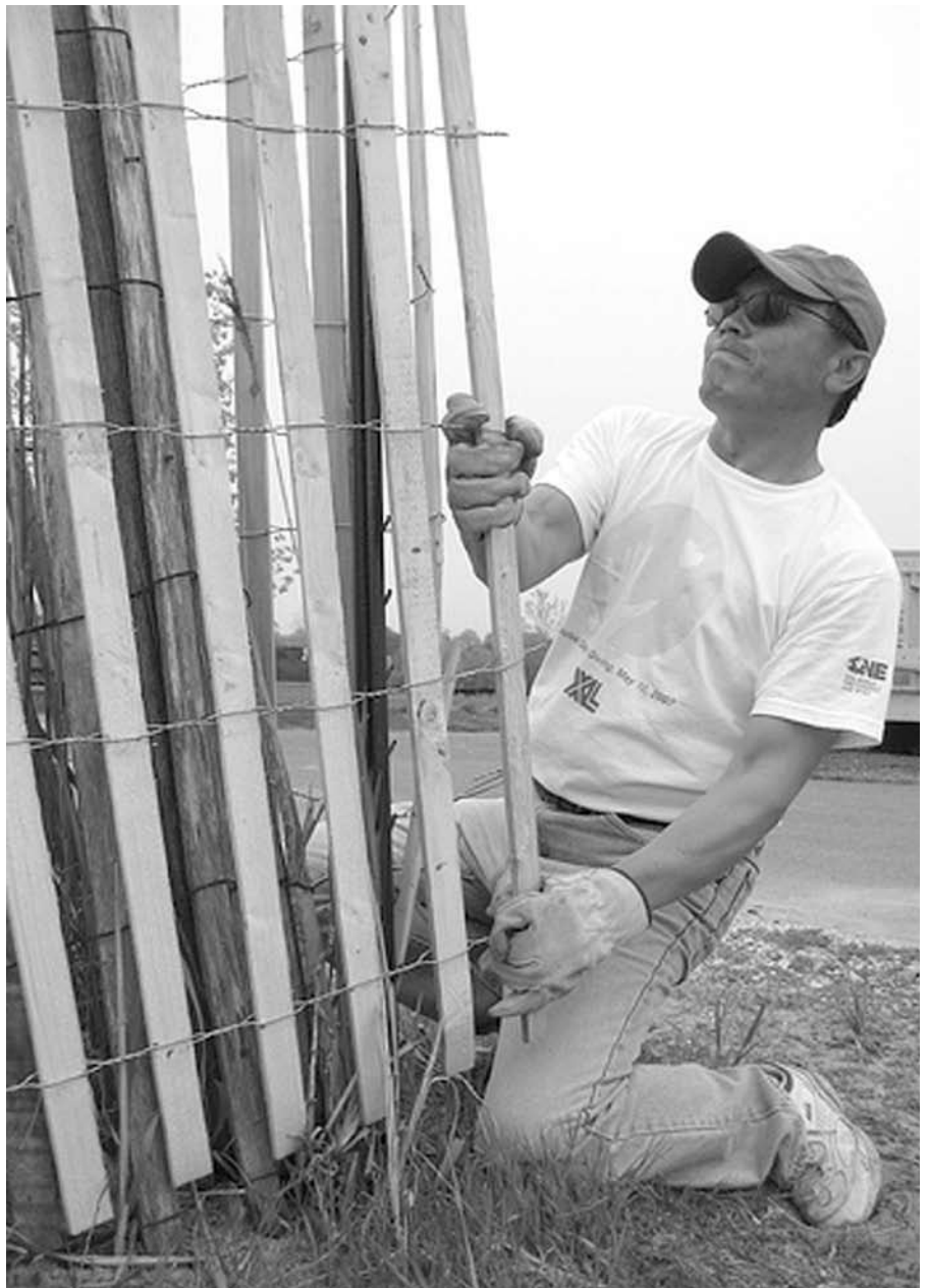
XL's Peter Chin makes repairs to a dune fence. Photos courtesy of XL.
