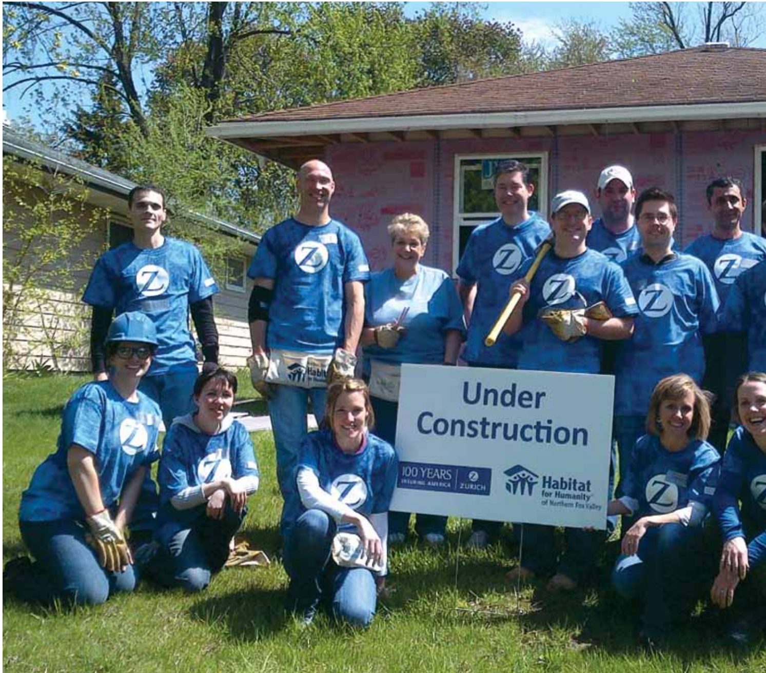
The Zurich team help Habitat for Humanity rebuild a home in Carpentersville, Illinois.
