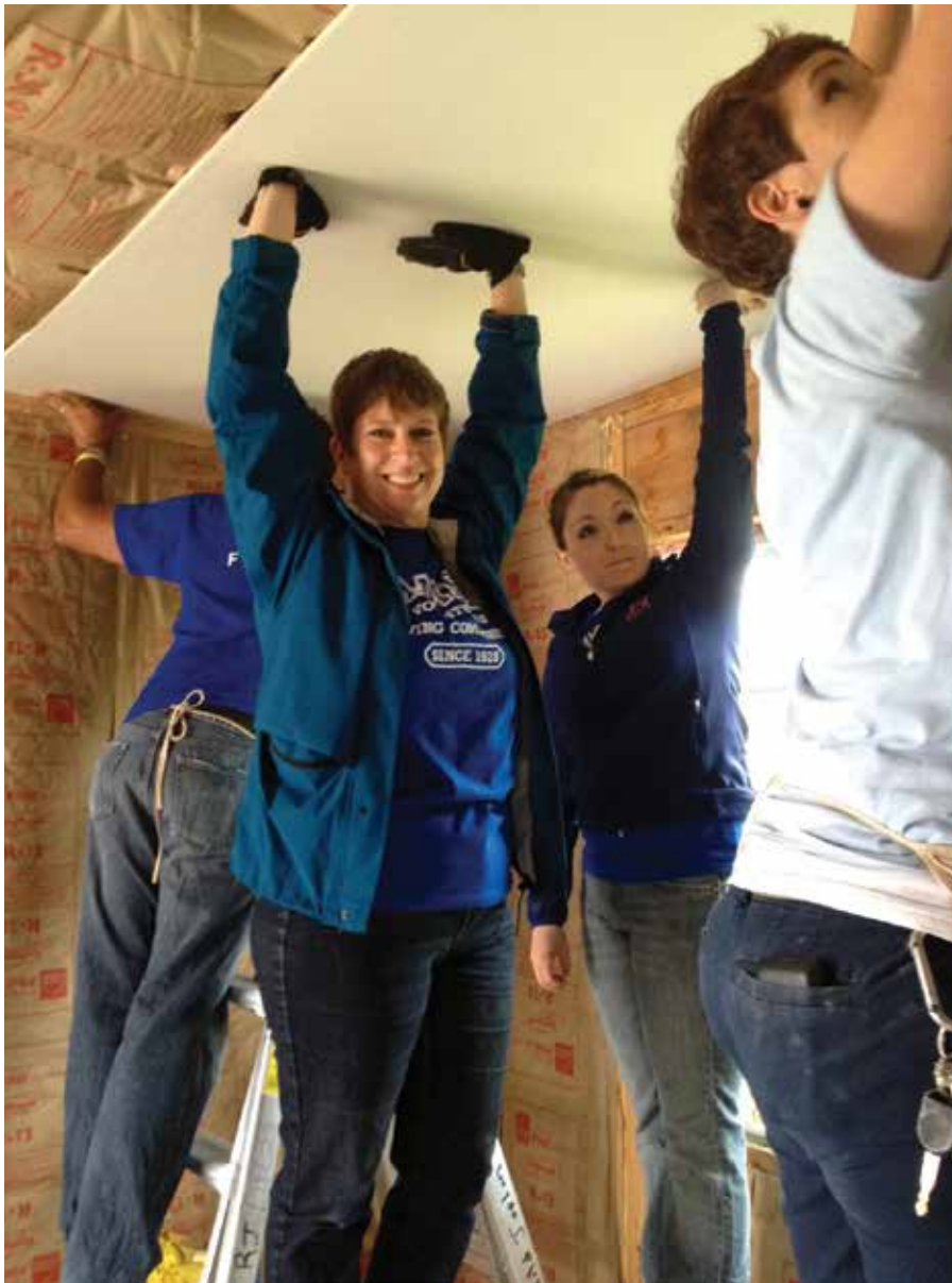
Volunteers from Farmers help hang drywall in a home in Joplin, Missouri.
